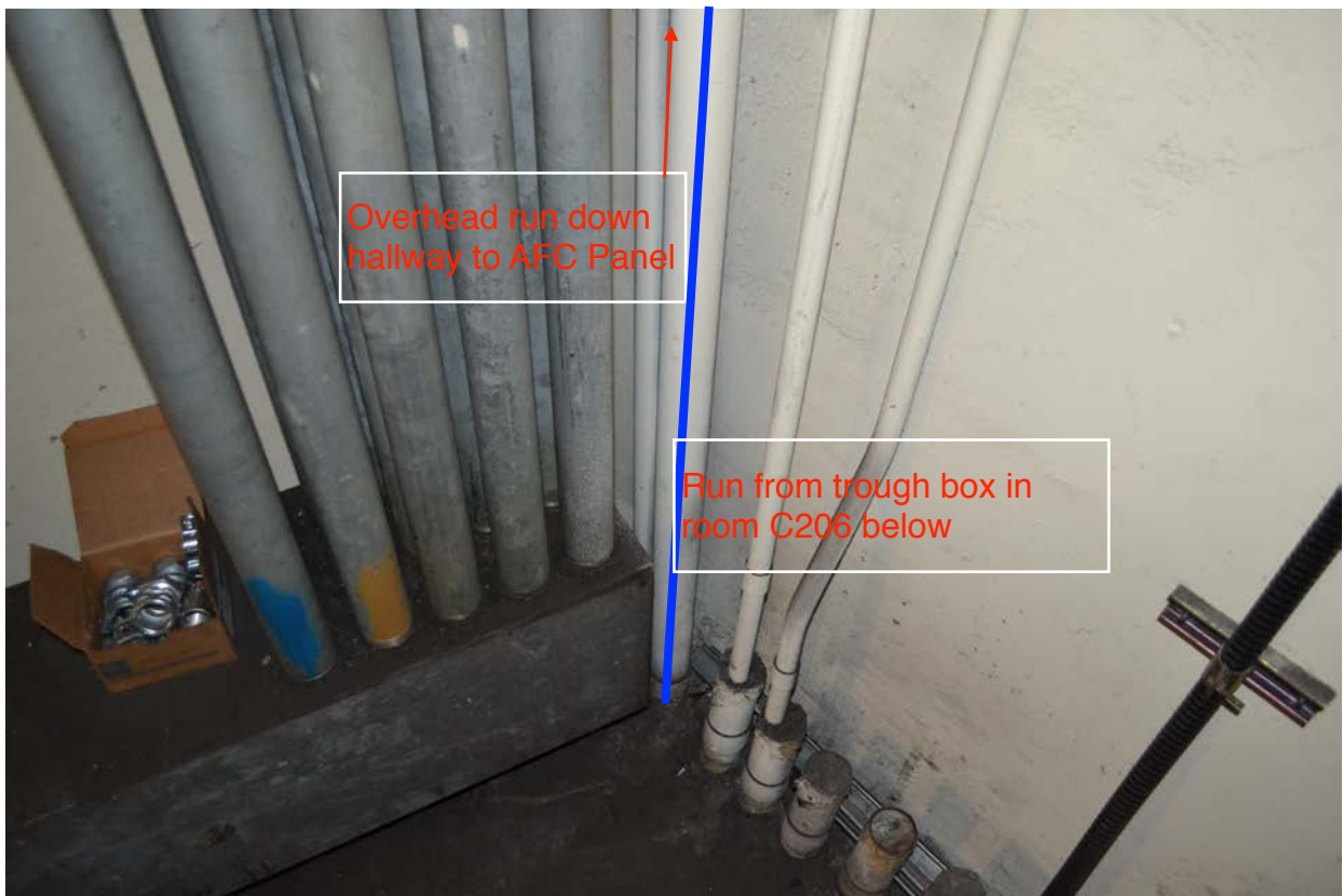
Photo #4 – C09 Crystal City: Conduit in room C300
