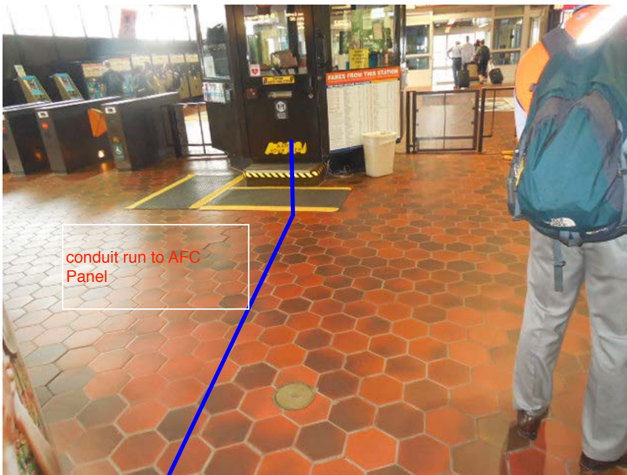
Photo #1 – C10 Reagan Airport South: Existing conduit run from Kiosk towards AFC Panel
