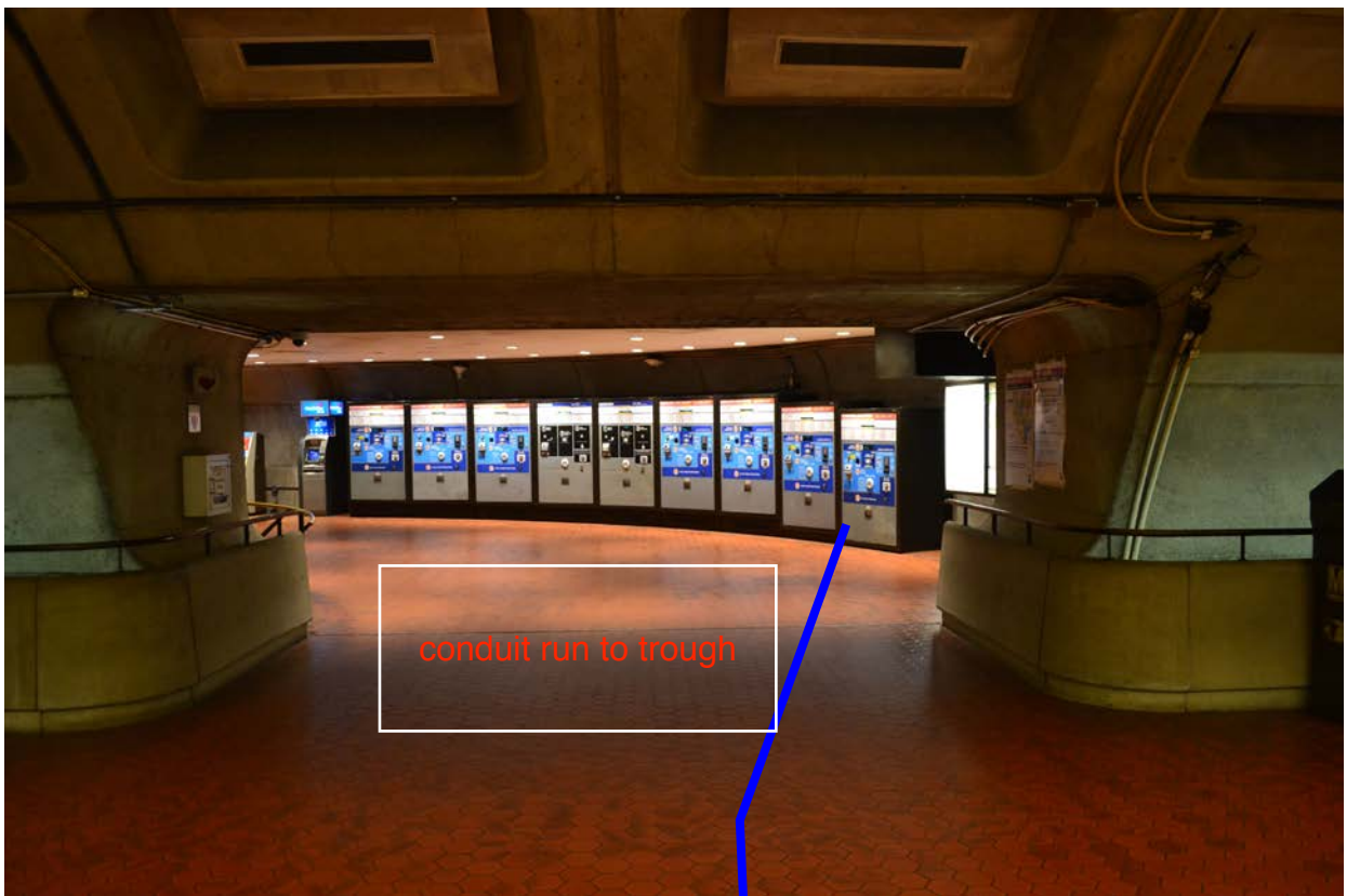
Photo #2 – C09 Crystal City: Power run from kiosk into trough box in room C206
